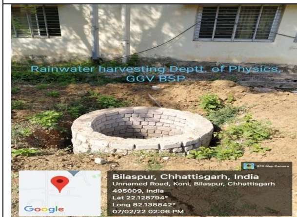
Rain Water Harvesting @ Physics Department
