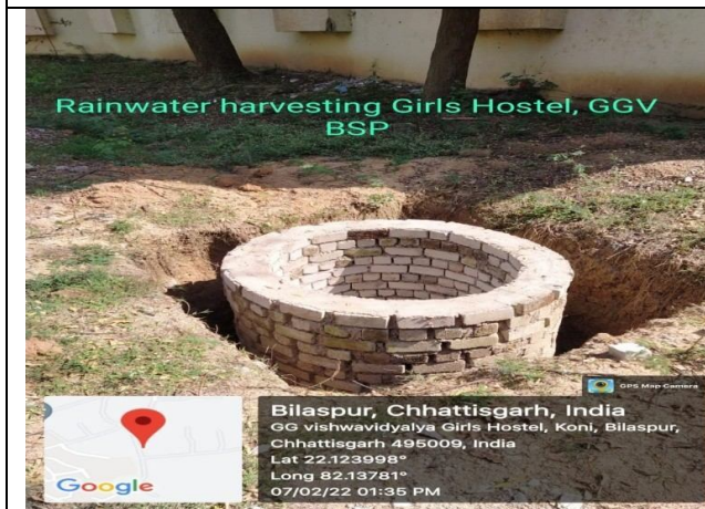
Rain Water Harvesting Girls Hostel
