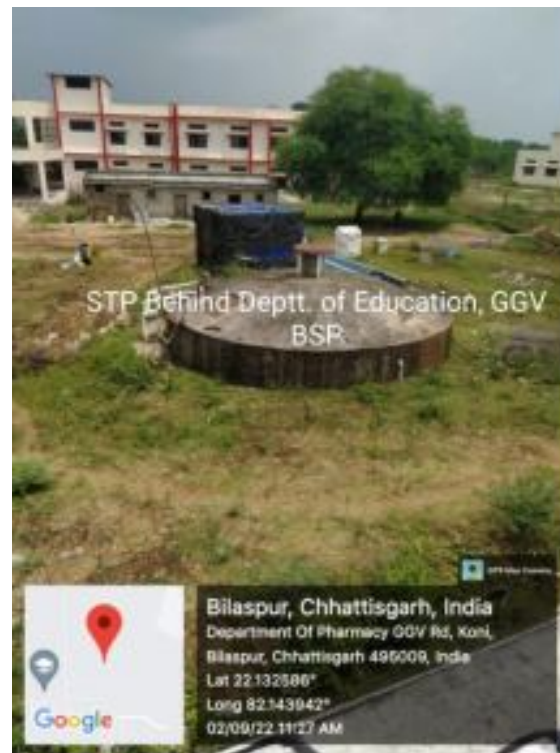
STP behind Department of Education
