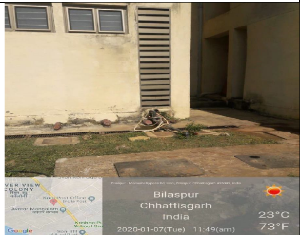
Rain Water Harvesting @ New Boys Hostel - A
