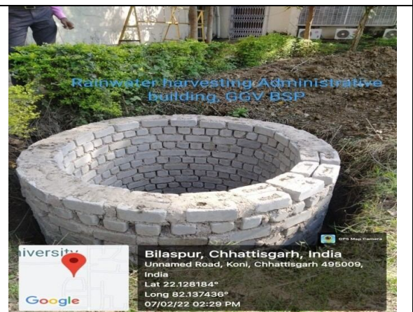
Rain Water Harvesting @ Administrative Building
